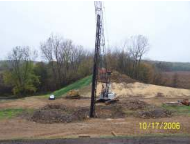
“Driving” the pilings for the foundations of the structures for the new bridge. (28 steel beams, 40 to 50 foot long)
