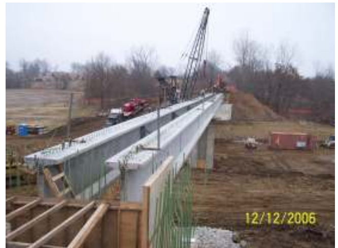
All four beams are in place now, and no, it’s not going to be a two-lane bridge. The next step is to form and pour a 10’ wide deck over the top of the beams.
