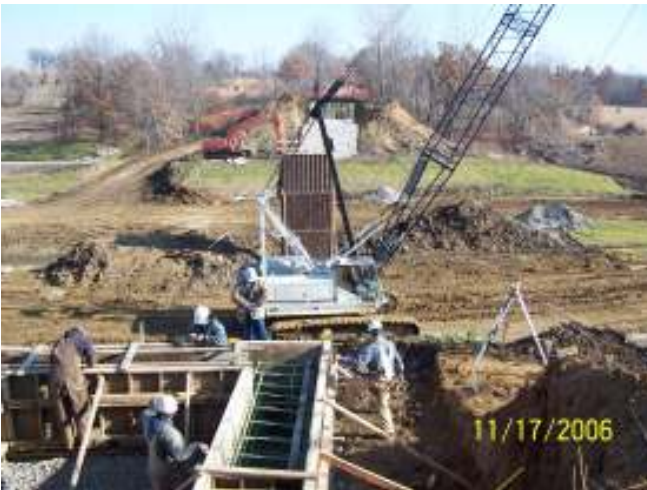
Building the structures that hold up the beams that hold up the bridge deck.
